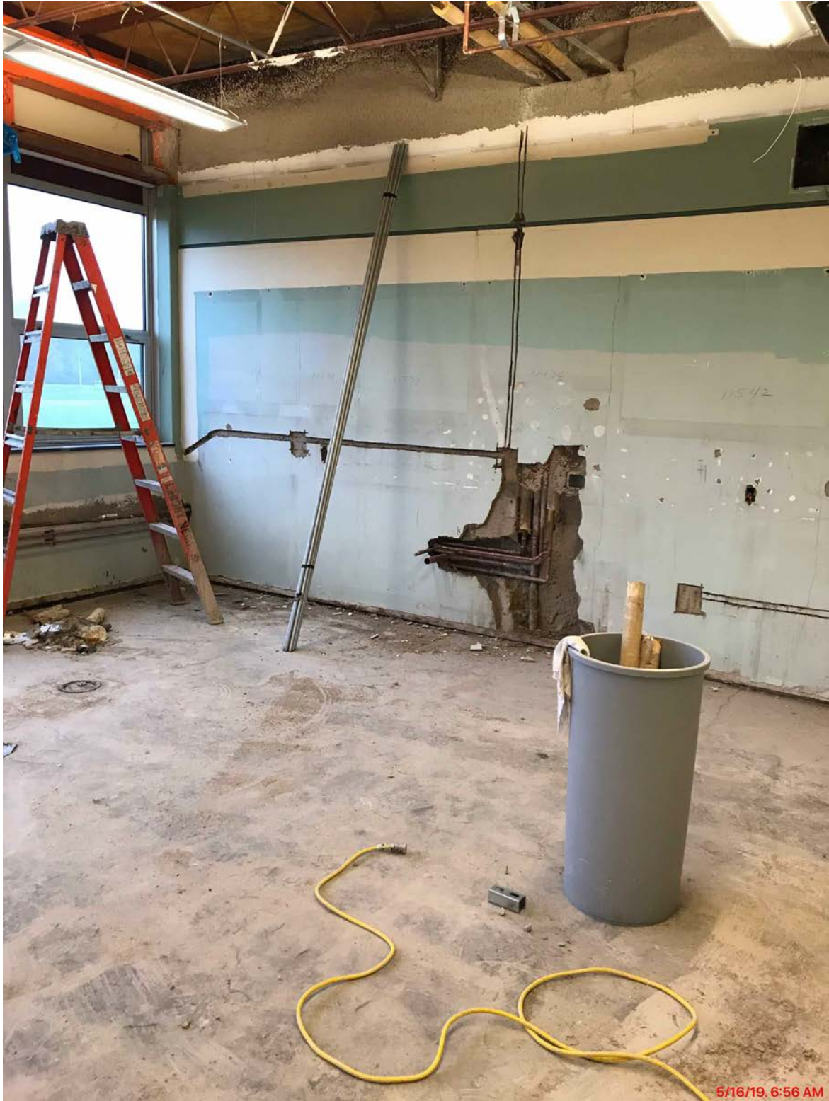
Underground Plumbing Installation Continues in Family and Consumer Science Room in HS/MS
