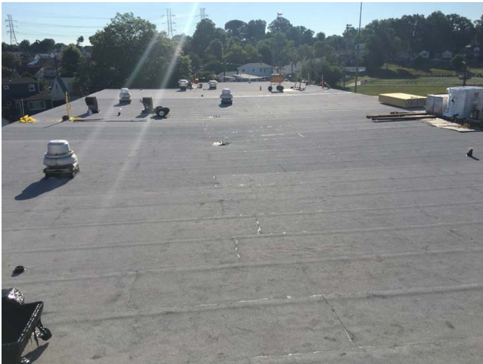
July 2018: Belleville HS – Cap Sheet installation substantially completed at HS Roof E
