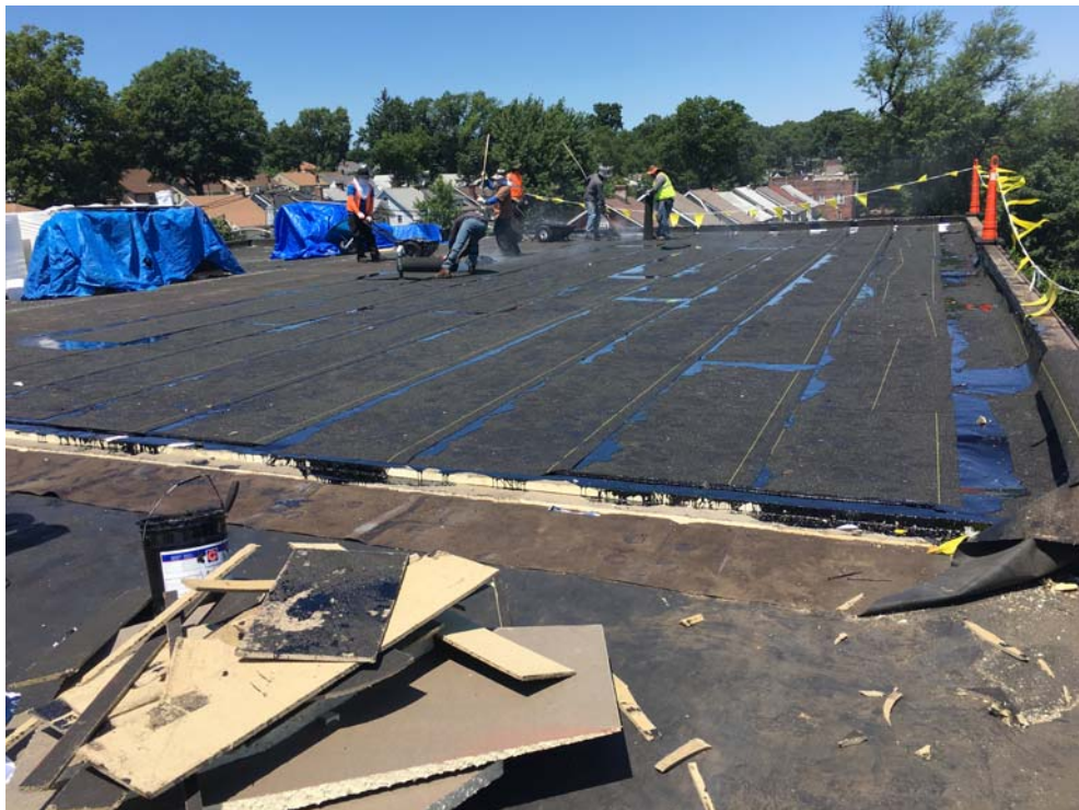
July 2018: Belleville ES #3 –Base sheet being installed in hot asphalt at Roof A2.
