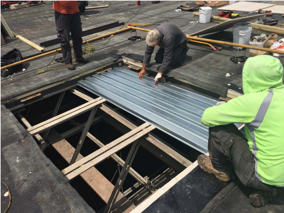
July 2018: Belleville HS – Deck infill at demolished abandoned existing mechanical equipment curb at HS Roof C.
