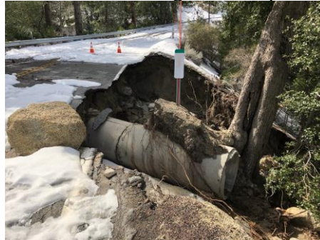
Newest wash out on SR 243.
