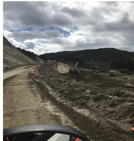
SR 74 near post mile 51 (unpaved segment of roadway with limited lane width).
