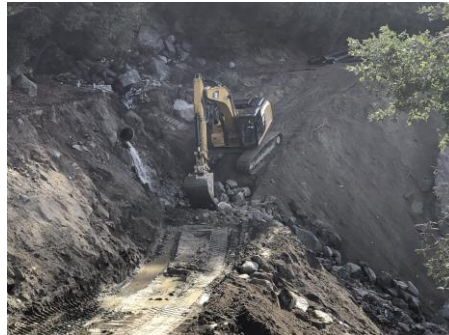
SR 243 near Lake Fulmor – running water impeding roadbed repair.
