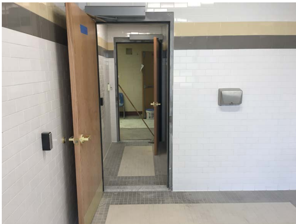
August 2018: Belleville HS – Wood door installation complete at 2nd floor Women’s Faculty Toilet.
