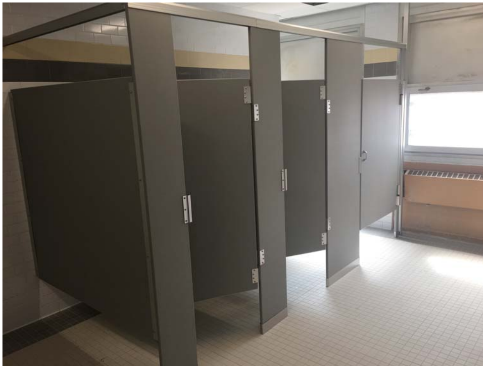
August 2018: Belleville HS – Toilet partitions installed in 2nd floor Girls' Student Toilet.
