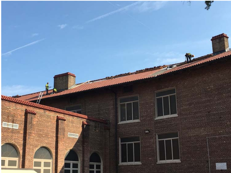
August 2018: Belleville ES #10 – Terra Cotta Roof Tiles being reinstalled following deck repairs.
