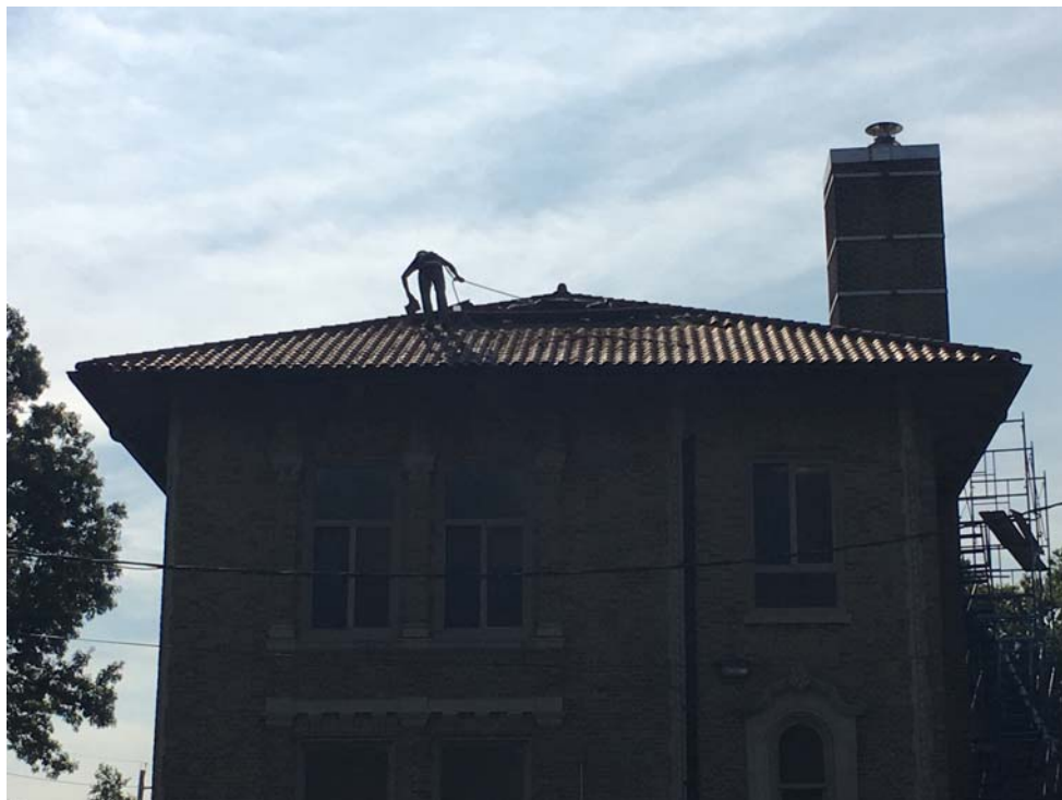
August 2018: Belleville ES #10 – Tiles being removed for deck inspection and underlayment installation.
