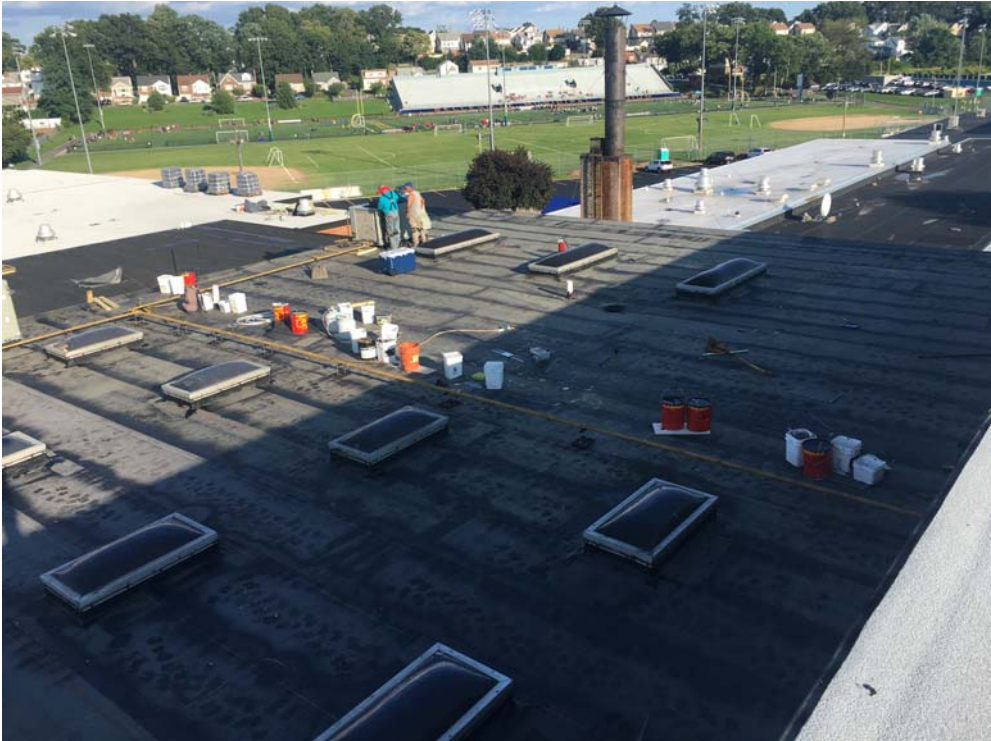
August 2018: Belleville HS – Roof replacement work completed on Roof B. Cap Sheet yet to be installed.
