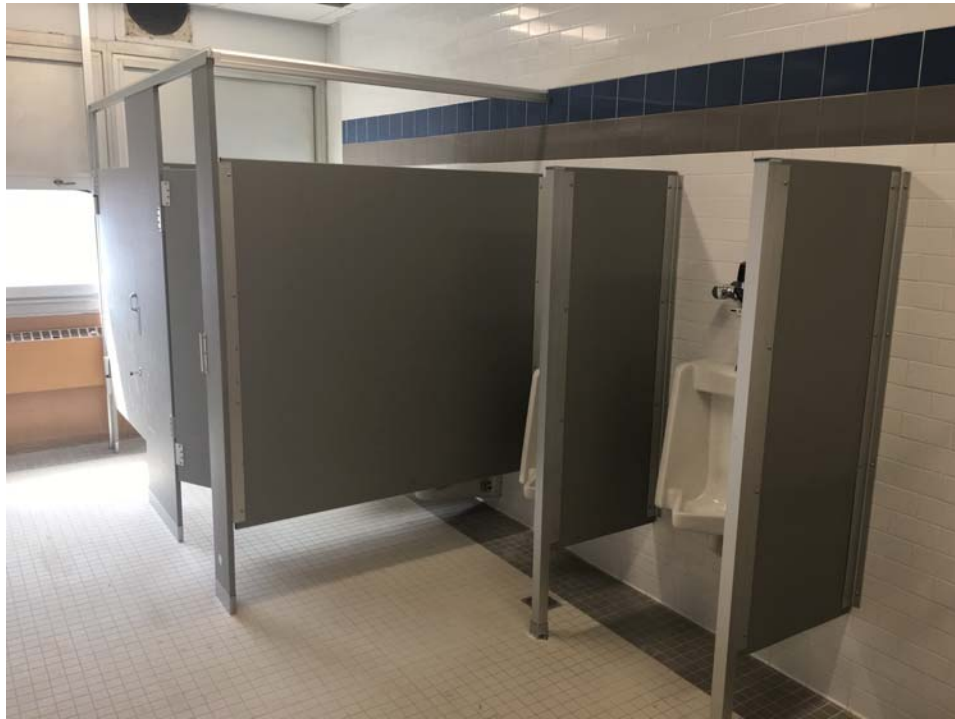
.August 2018: Belleville HS –Toilet partitions installed in 2nd floor Boys' Student Toilet.
