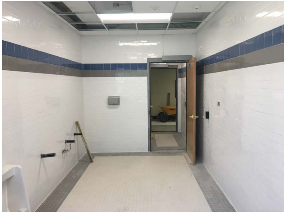
August 2018: Belleville HS – Wood door installation complete at 2nd floor Men’s Faculty Toilet.
