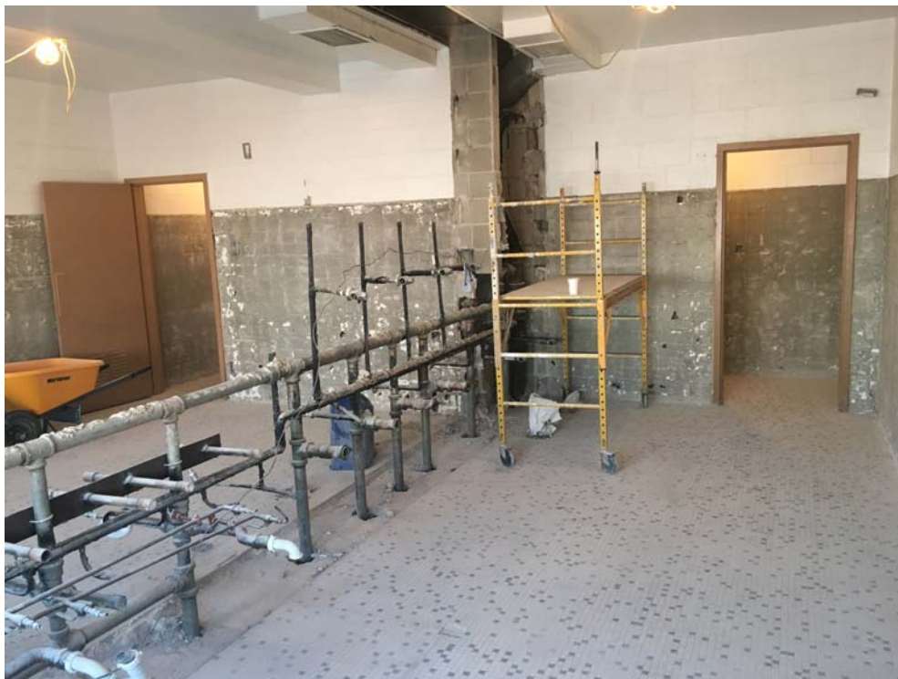
July 2018: Belleville HS – Ongoing demolition in high school 2 nd floor student toilets #206 & #208.
