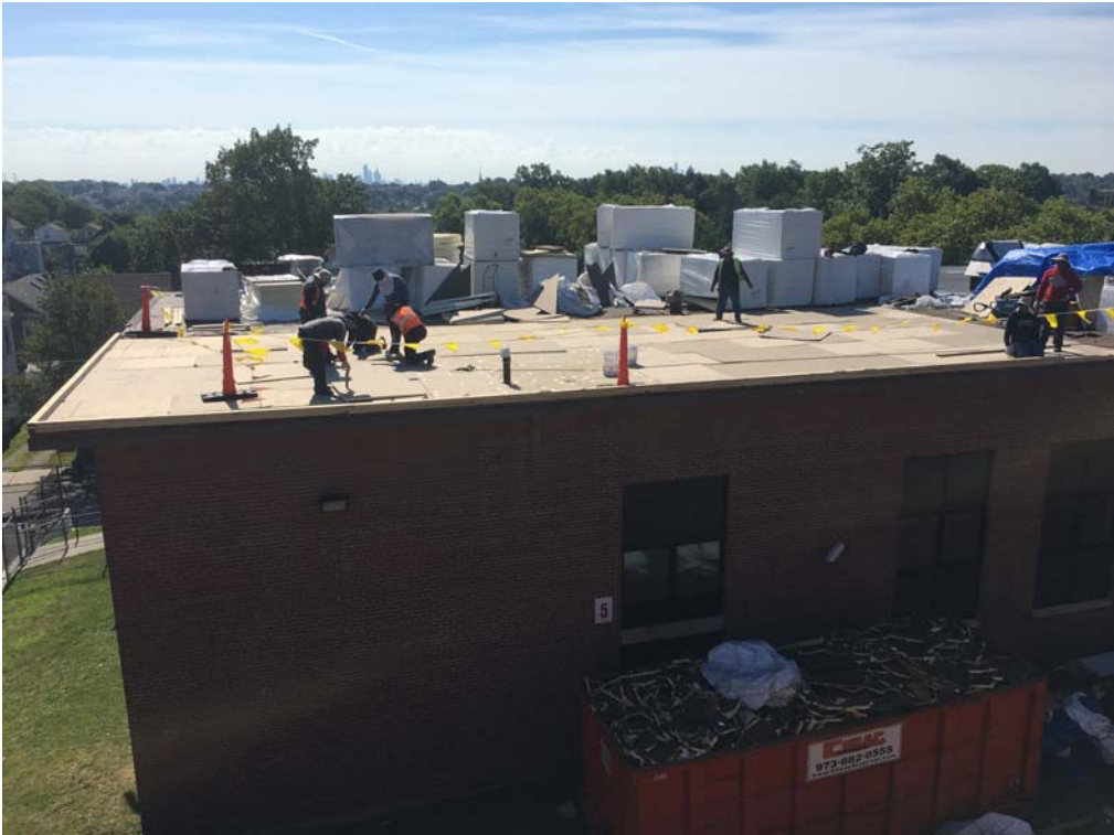
July 2018: Belleville ES #3 –Ongoing installation of new roof insulation at Roof C1.
