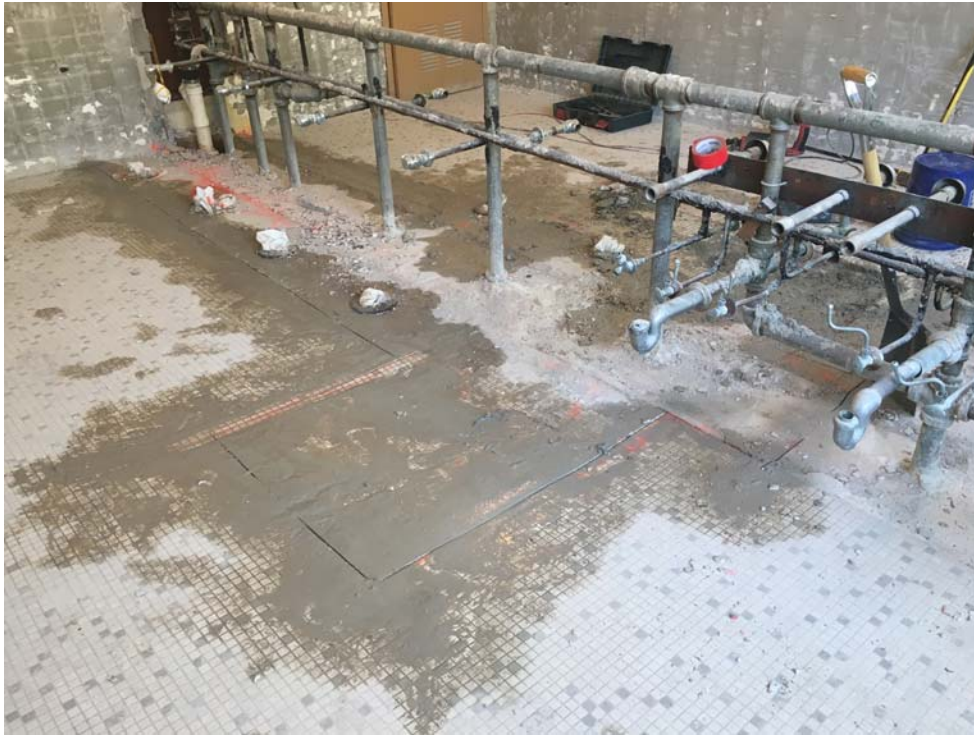
July 2018: Belleville HS –Ongoing demolition in high school 2nd floor Faculty Toilets #242 & #245.
