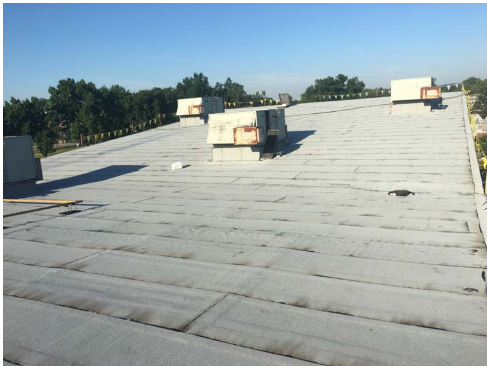
July 2018: Belleville HS – Cap Sheet installation substantially completed at HS Roof C.
