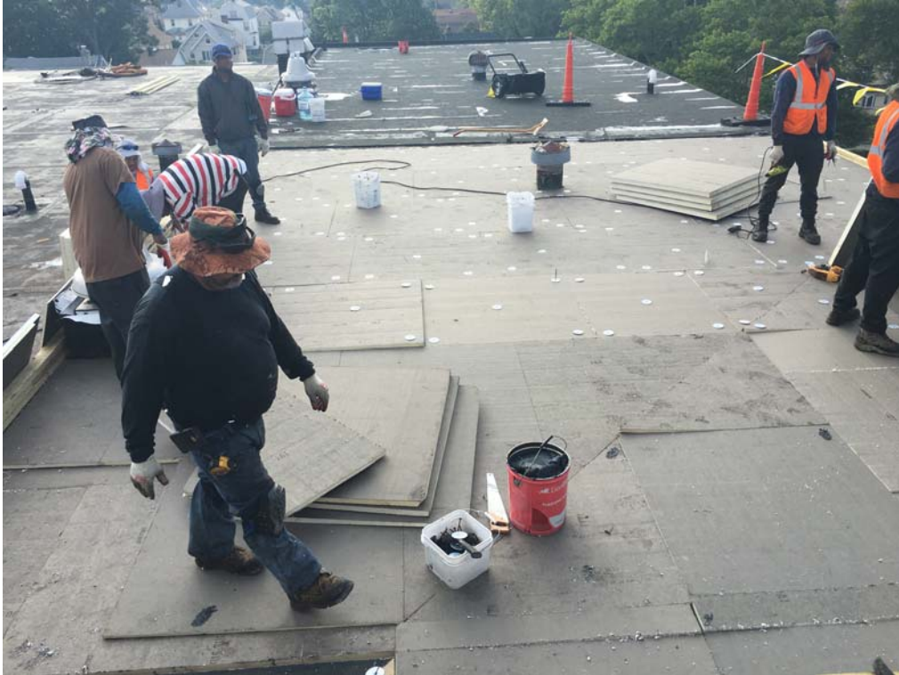
July 2018: Belleville ES #3– Ongoing installations of new roof insulation at Roof B.
