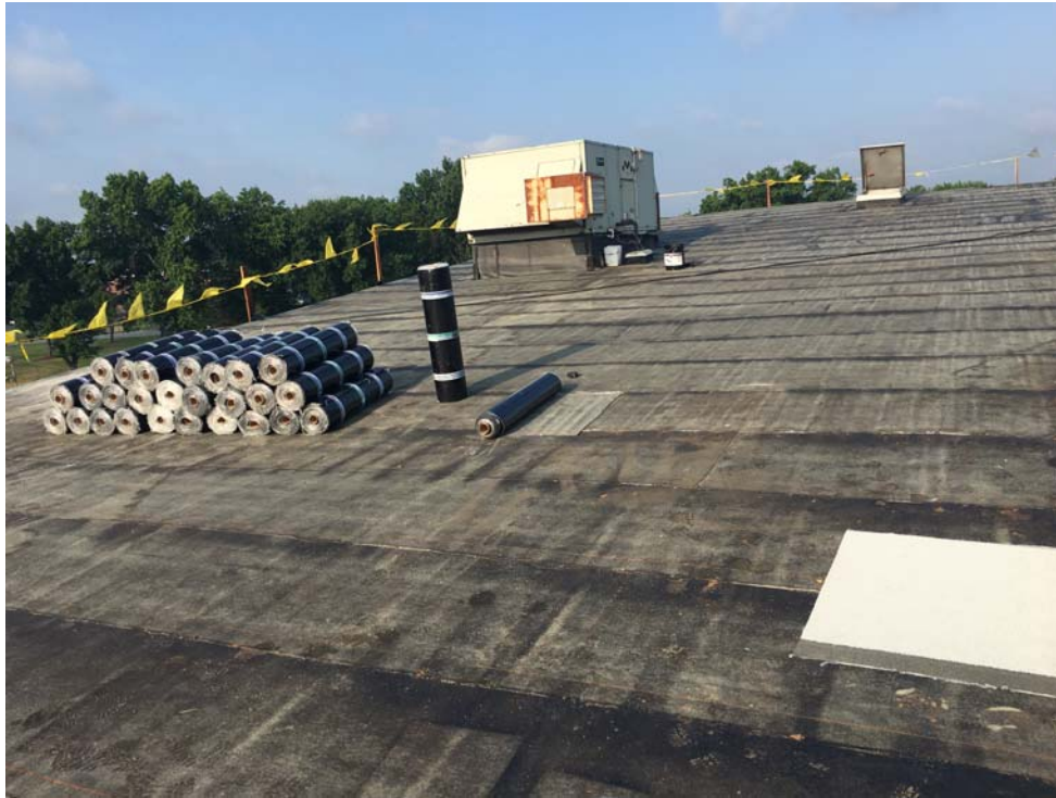
July 2018: Belleville HS – Completed torch applied base sheets at high school Roof C.
