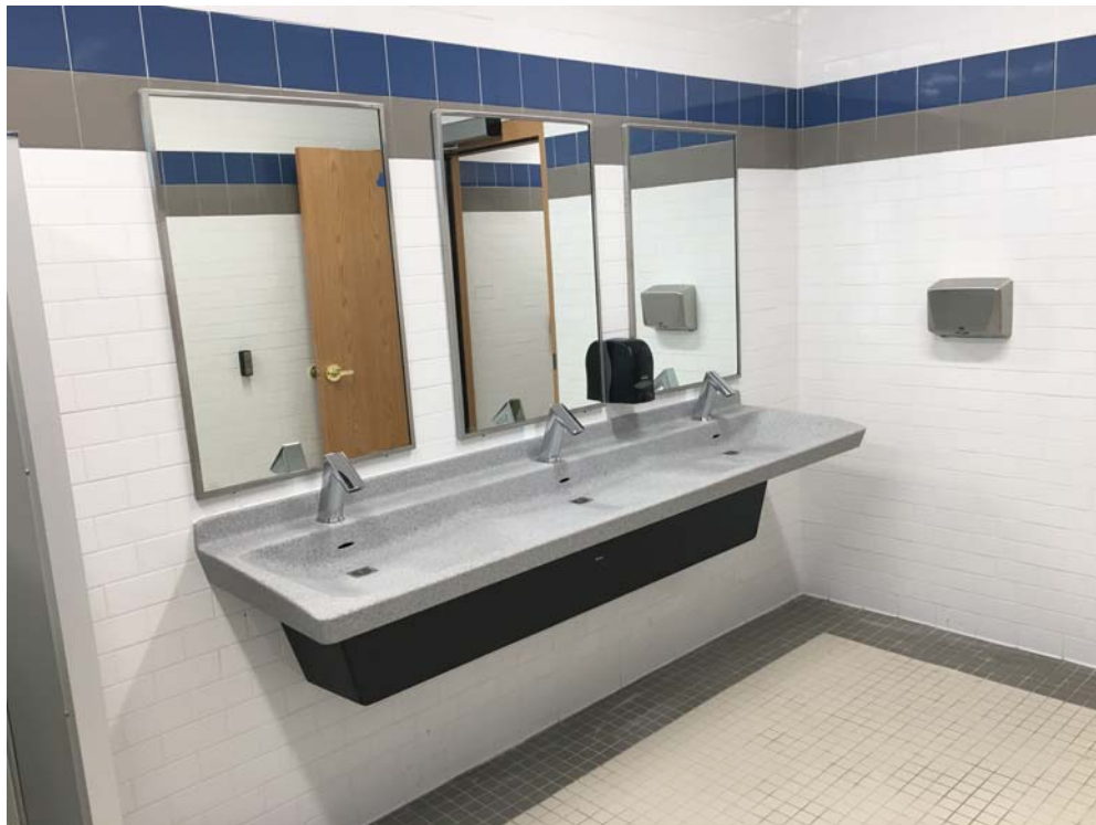
August 2018: Belleville HS – Sink & bathroom accessories installed in 2nd floor Men’s Faculty Toilet.
