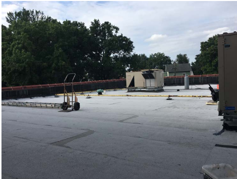
August 2018: Belleville ES #10 – Roof replacement work substantially completed on the sole flat roof.
