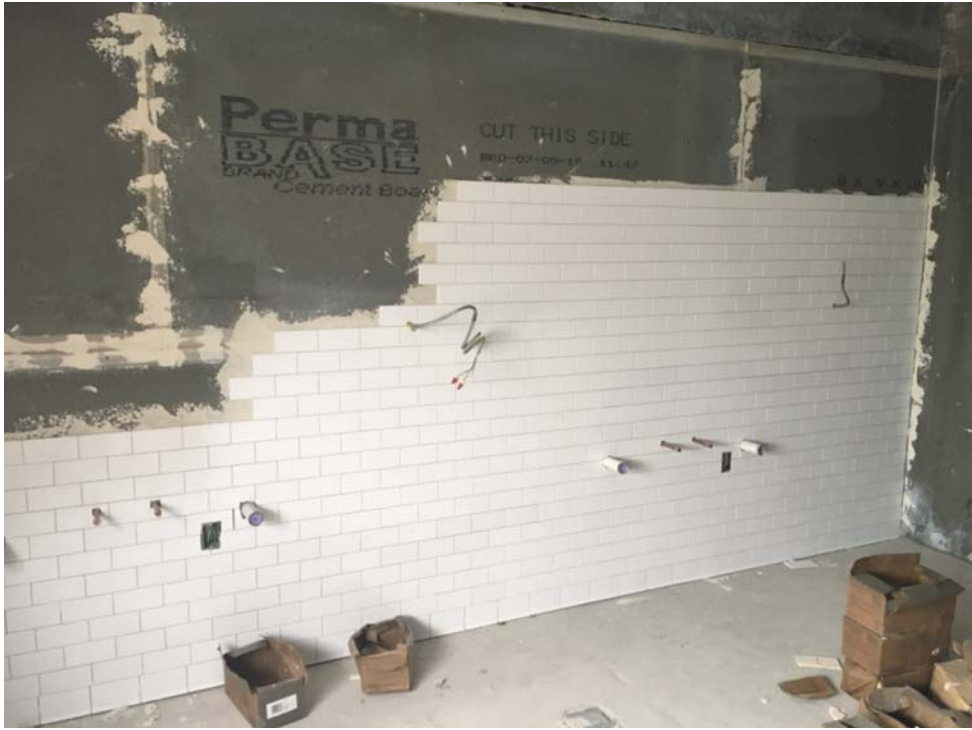
August 2018: Belleville HS – Ongoing Ceramic wall tile installation in 1 st floor Girls' Toilet.
