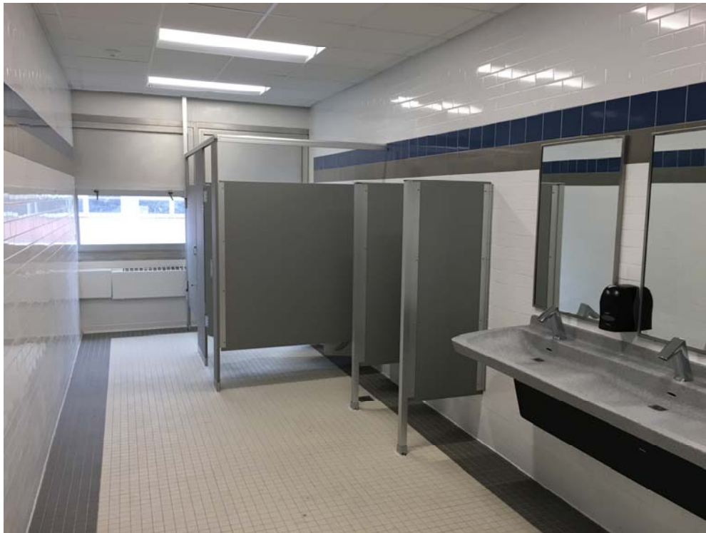
.August 2018: Belleville HS –Sink & bathroom accessories installed in 2nd floor Boys' Student Toilet.
