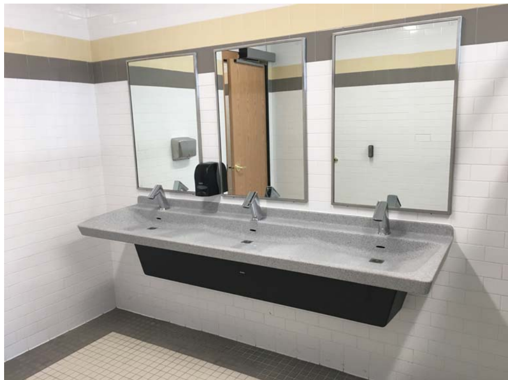
August 2018: Belleville HS – Sink & bathroom accessories installed in 2nd floor Women’s Faculty Toilet.
