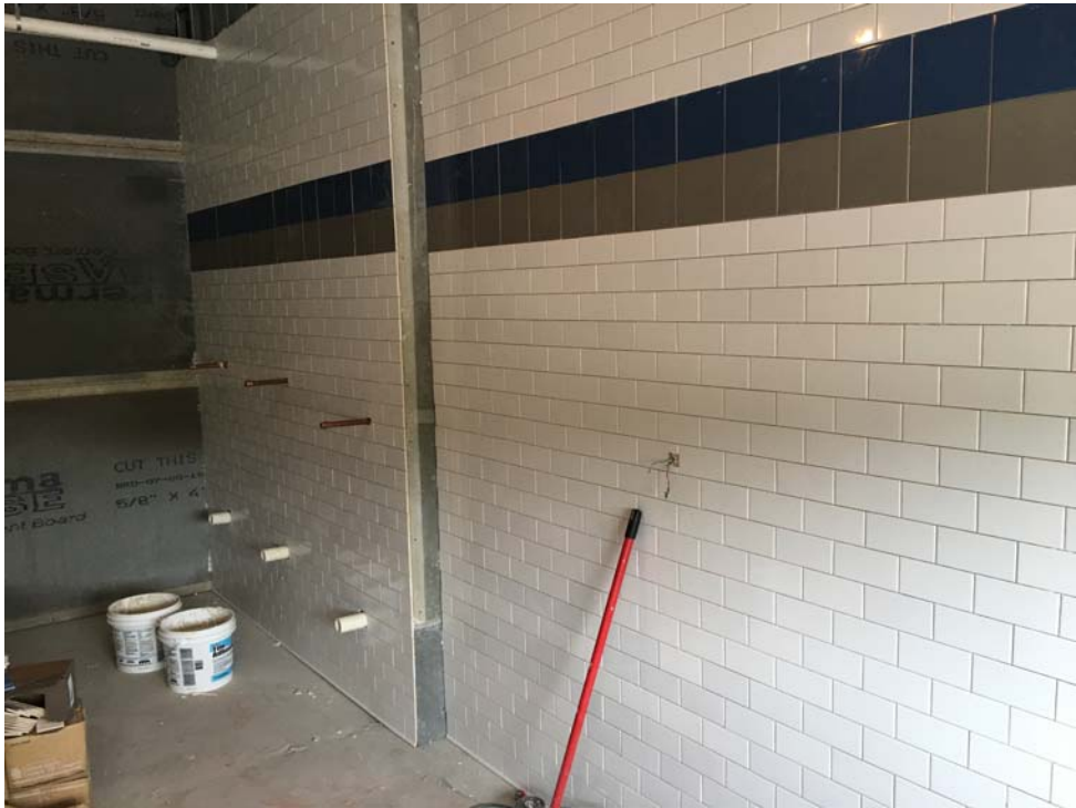
August 2018: Belleville HS – Ongoing Ceramic wall tile installation in 1 st floor Boys' Toilet.
