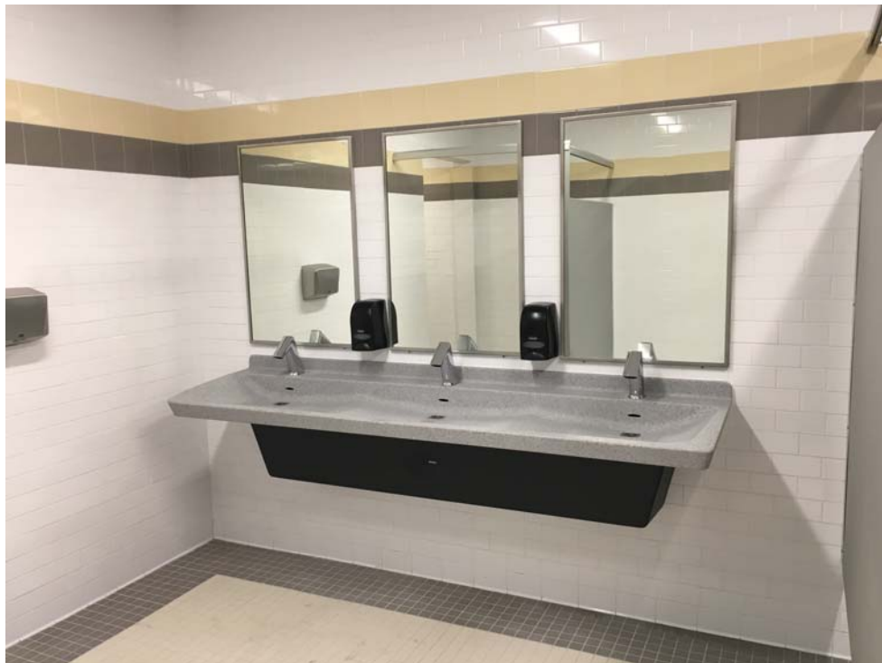
August 2018: Belleville HS – Sink & bathroom accessories installed in 2nd floor Girls' Student Toilet.
