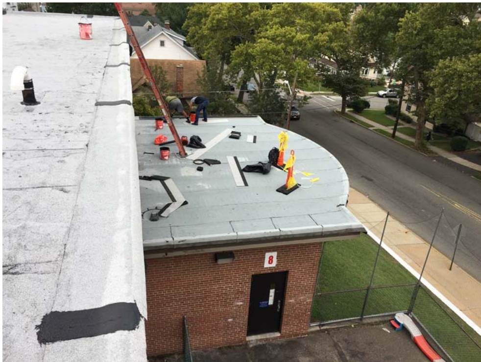
September 2018: Belleville ES #3 – Preparation for perimeter trims installation at low radius roof.
