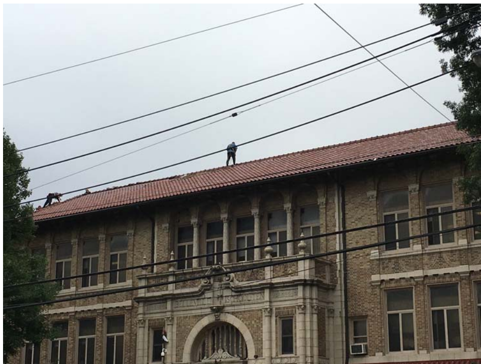
September 2018: Belleville ES #10 – Tile removals and deck inspection at the final area of Terra Cotta Roof Tile work being completed at ES #10
