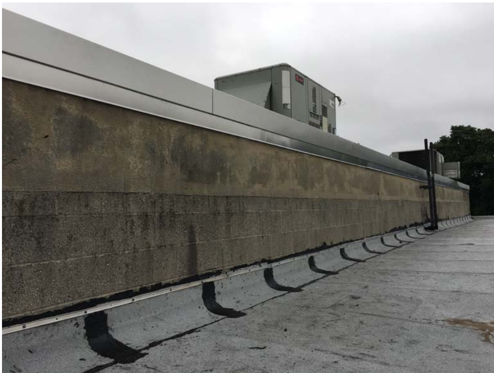
September 2018: Belleville HS – Completed perimeter trim and flashing work at Roof A.
