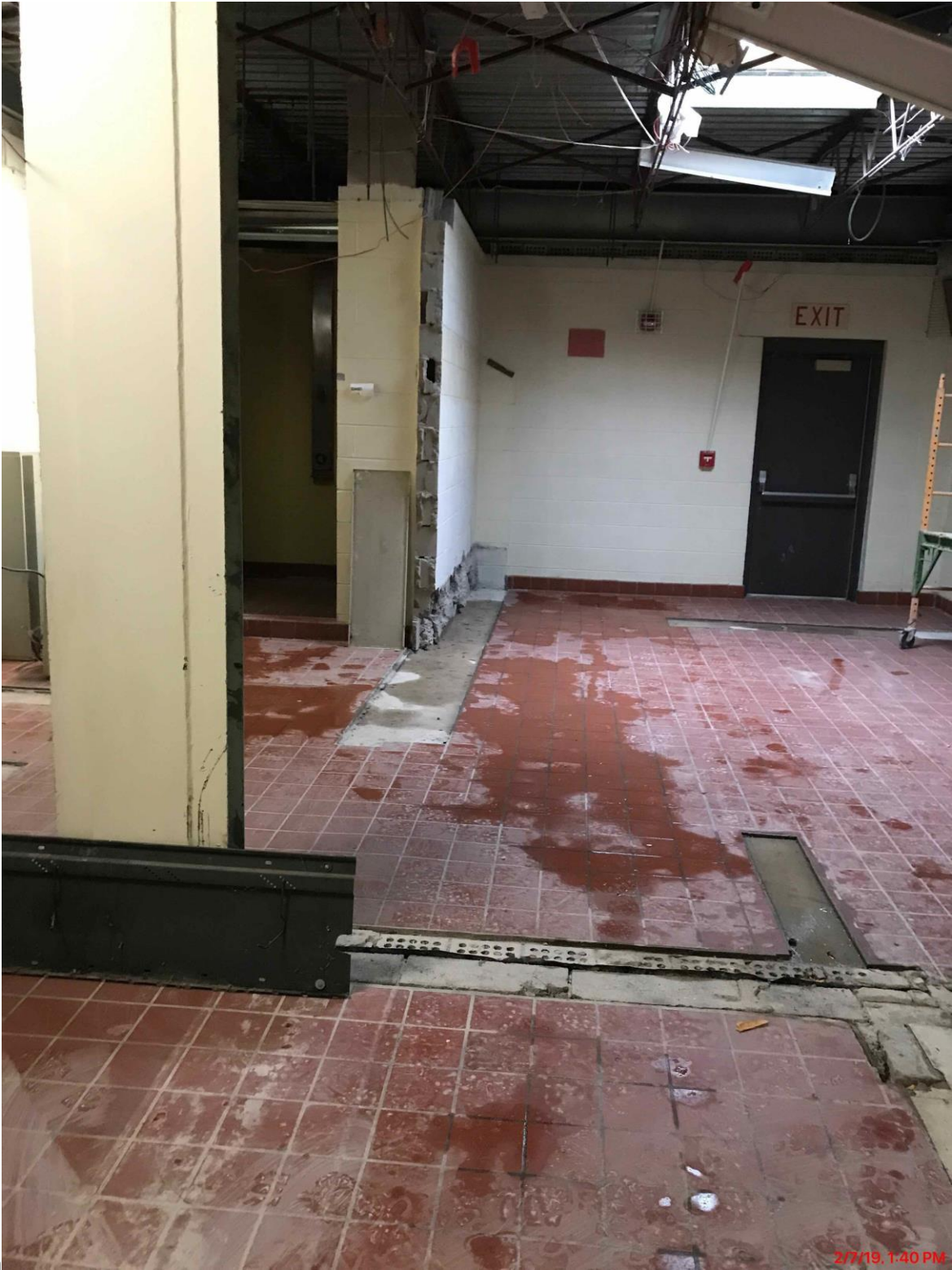
Finishing Up Pre Abatement Demolition in Elementary Girls Locker Room/ P.E. Office.
