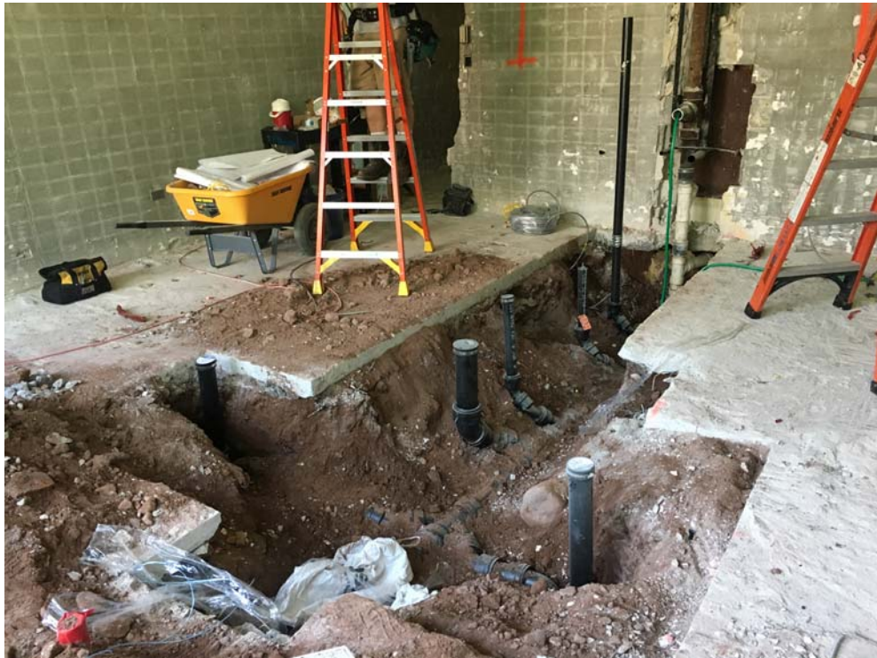
July 2018: Belleville HS –Below slab plumbing rough-ins at 2nd floor Faculty Toilets #242 & #245.
