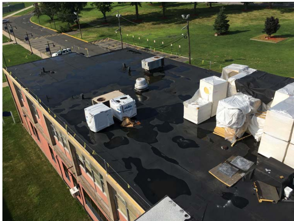
July 2018: Belleville HS – Perimeter protection installed in preparation for start of roofing at Roof D2.
