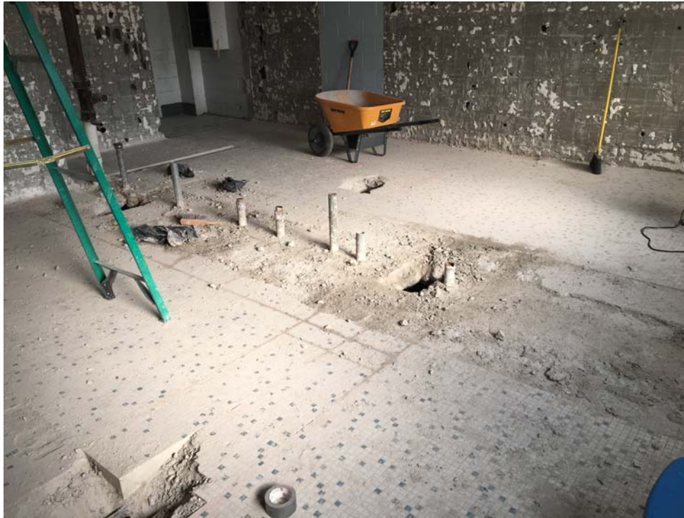
July 2018: Belleville HS –Ongoing demolition in high school 1 st floor student toilets #137 & #138.
