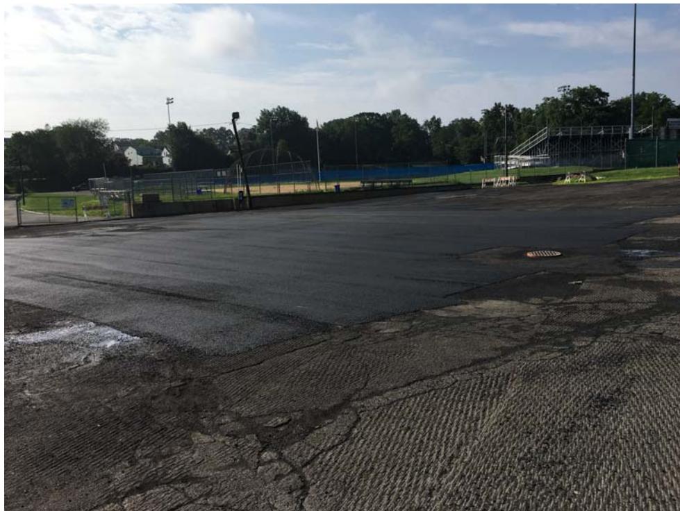
July 2018: Belleville HS – Leveling course of asphalt installed at high school parking lot.
