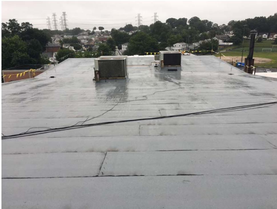
July 2018: Belleville HS – Completed base sheet installation at high school Roof C.
