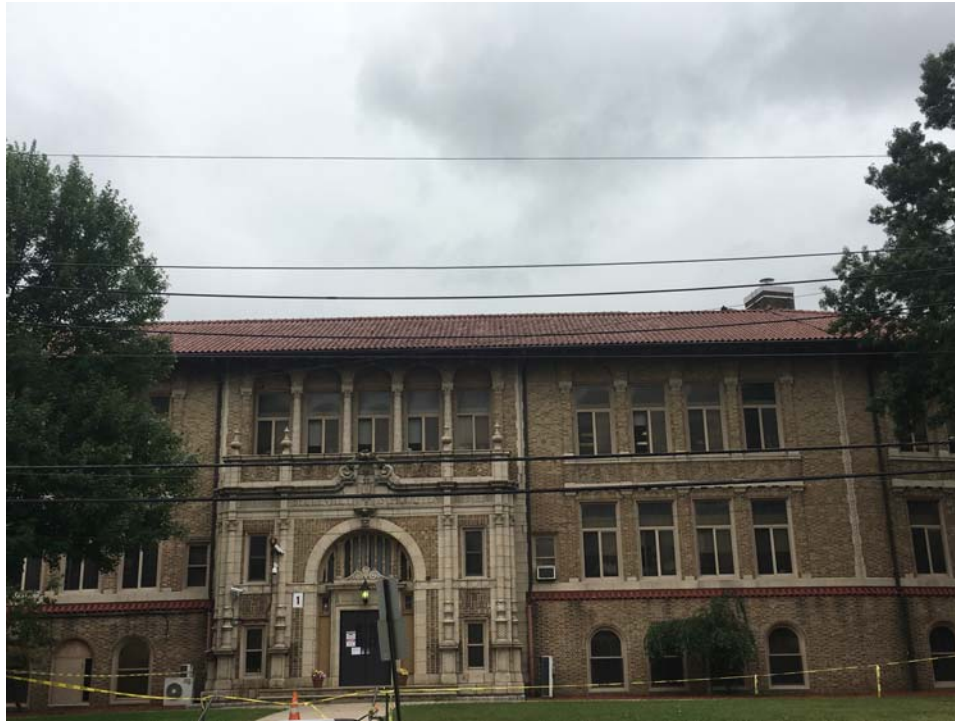
September 2018: Belleville ES #10 – Tile removals, deck inspection & underlayment installations completed at ES #10
