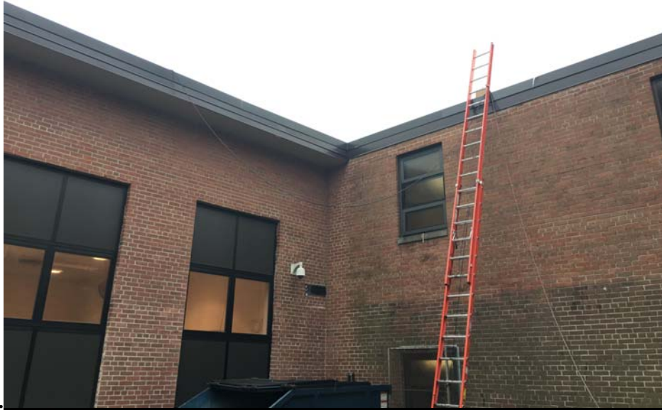
September 2018: Belleville ES #3 – Metal perimeter trims (fascia extensions) installation completed at Roof C1 and C2.
