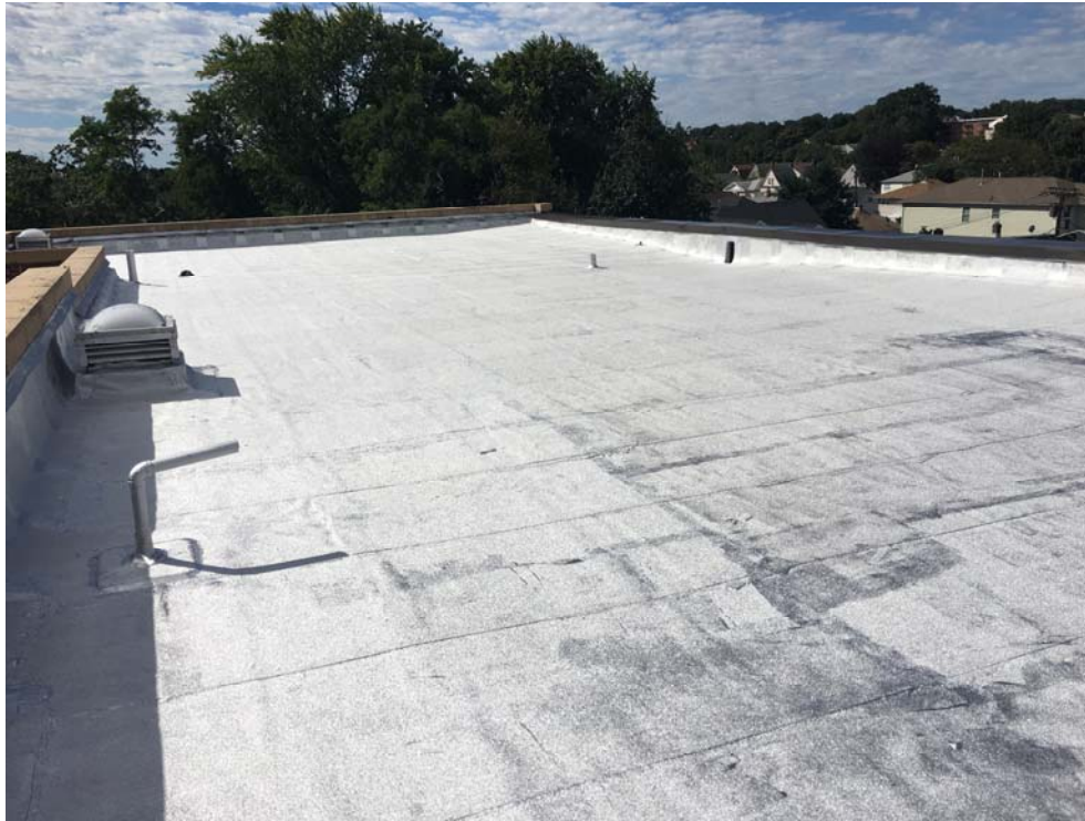
September 2018: Belleville ES #9 – Roof coating application (first coat) at ES #9 Roof B.
