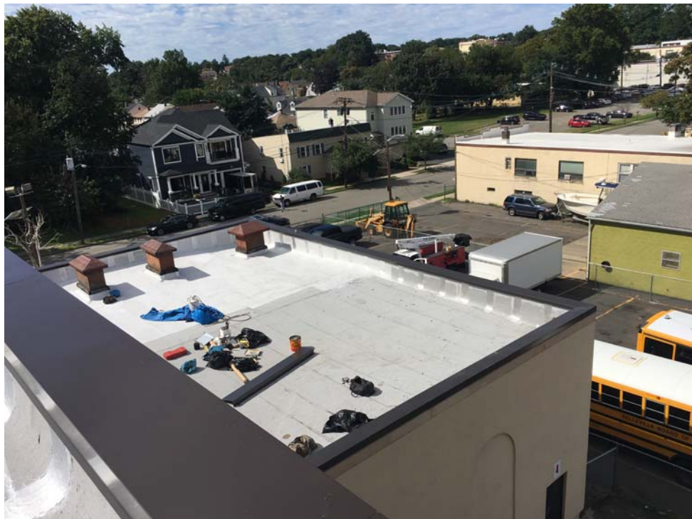
September 2018: Belleville ES #9 – Ongoing roof coating application (first coat) at ES #9 Roof A.
