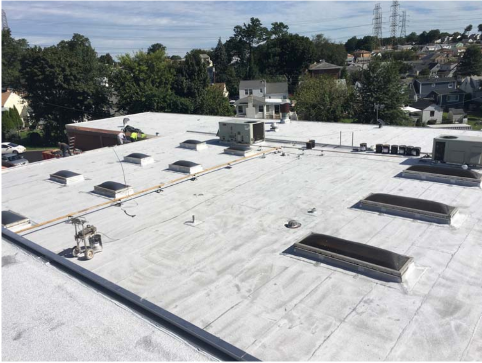
September 2018: Belleville HS – Roof coating application (first coat) at high school Roof B.
