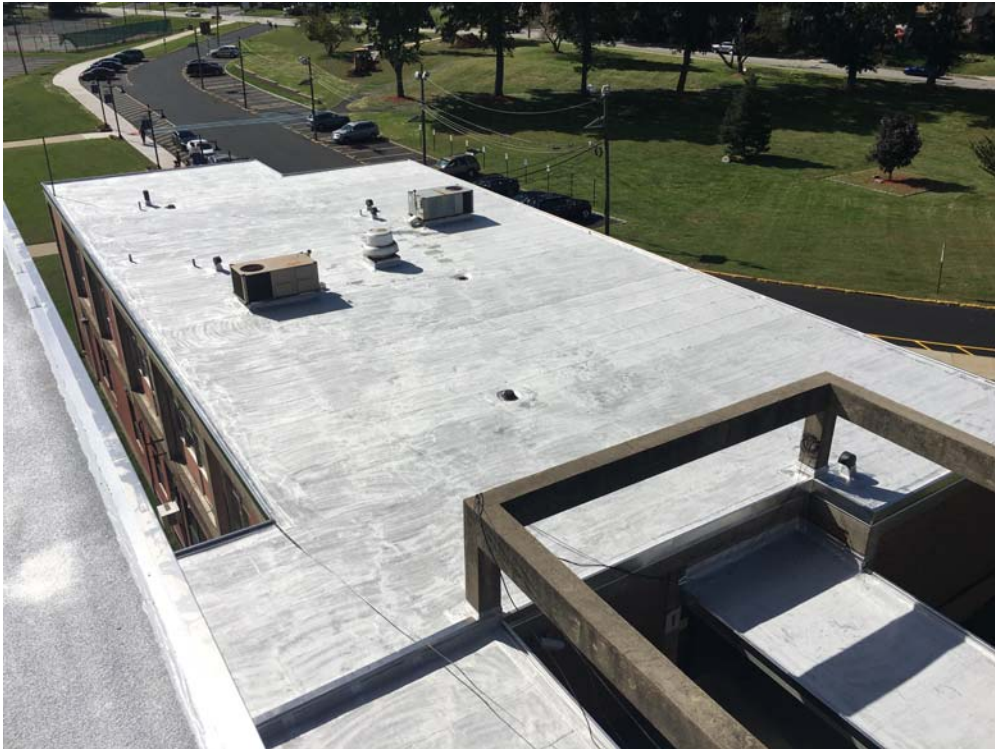
September 2018: Belleville HS – Roof coating application (first coat) at high school Roof D2.
