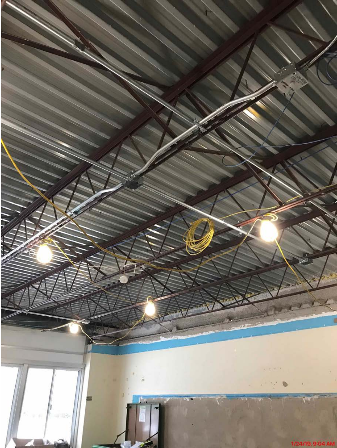
Upgrading Electrical and Installation of Enhanced Data Capabilities Continues - Eight Elementary Classrooms
