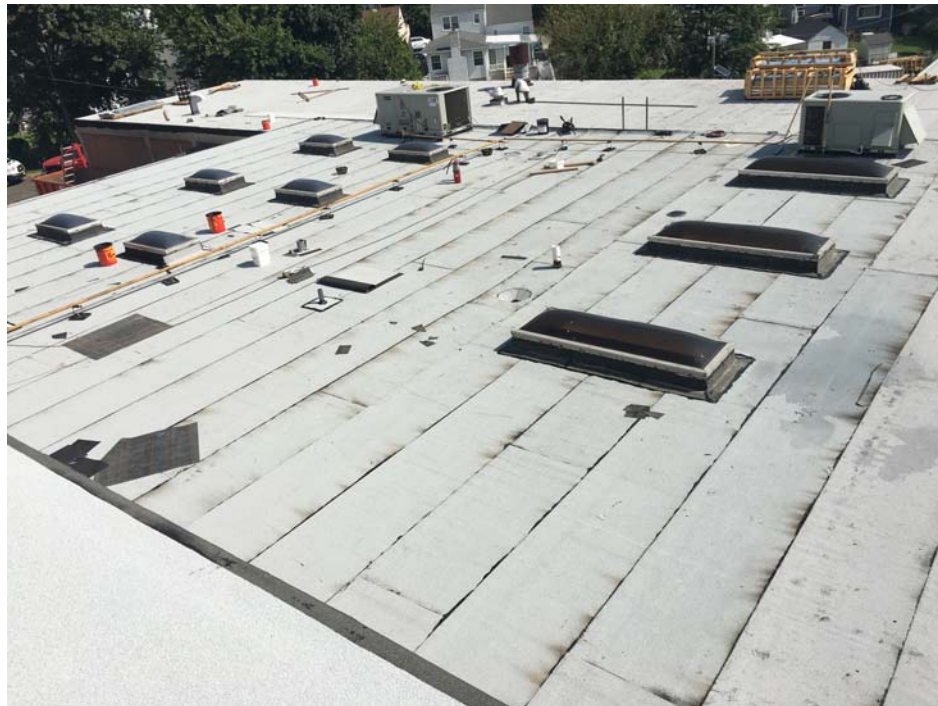
September 2018: Belleville HS – Completed Cap sheet installation at Roof B; the final area of roof replacement work.
