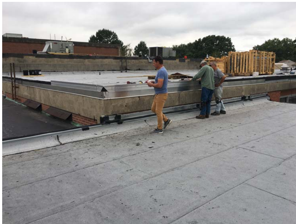
September 2018: Belleville HS – Ongoing metal perimeter trim installation at HS Roof A.
