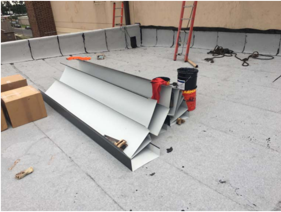
September 2018: Belleville ES #9 – Perimeter trims (copings) delivered and hoisted up to roof.
