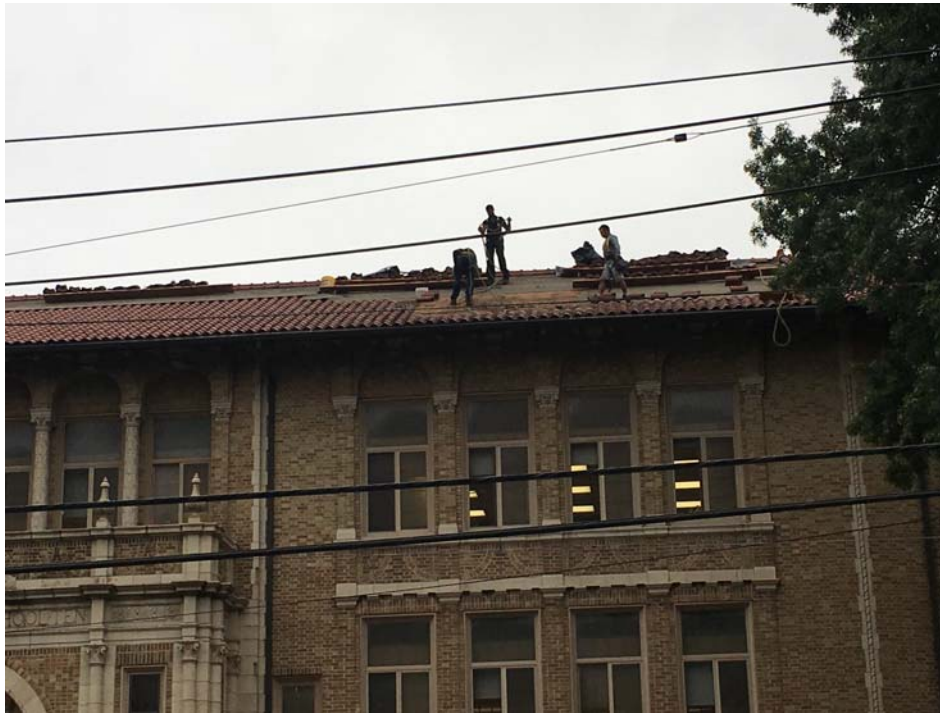
September 2018: Belleville ES #10 – Tile removals and deck inspection at the final area of Terra Cotta Roof Tile work commences at ES #10.
