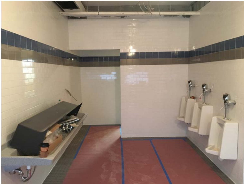
September 2018: Belleville HS – Ceramic wall and floor tile completed in 1 st floor Boys' Toilet.
