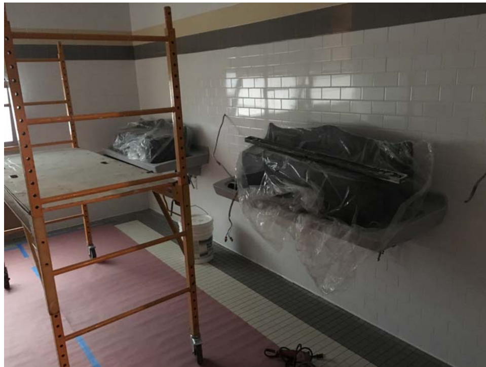
September 2018: Belleville HS – Ceramic wall and floor tile completed in 1 st floor Girls' Toilet.
