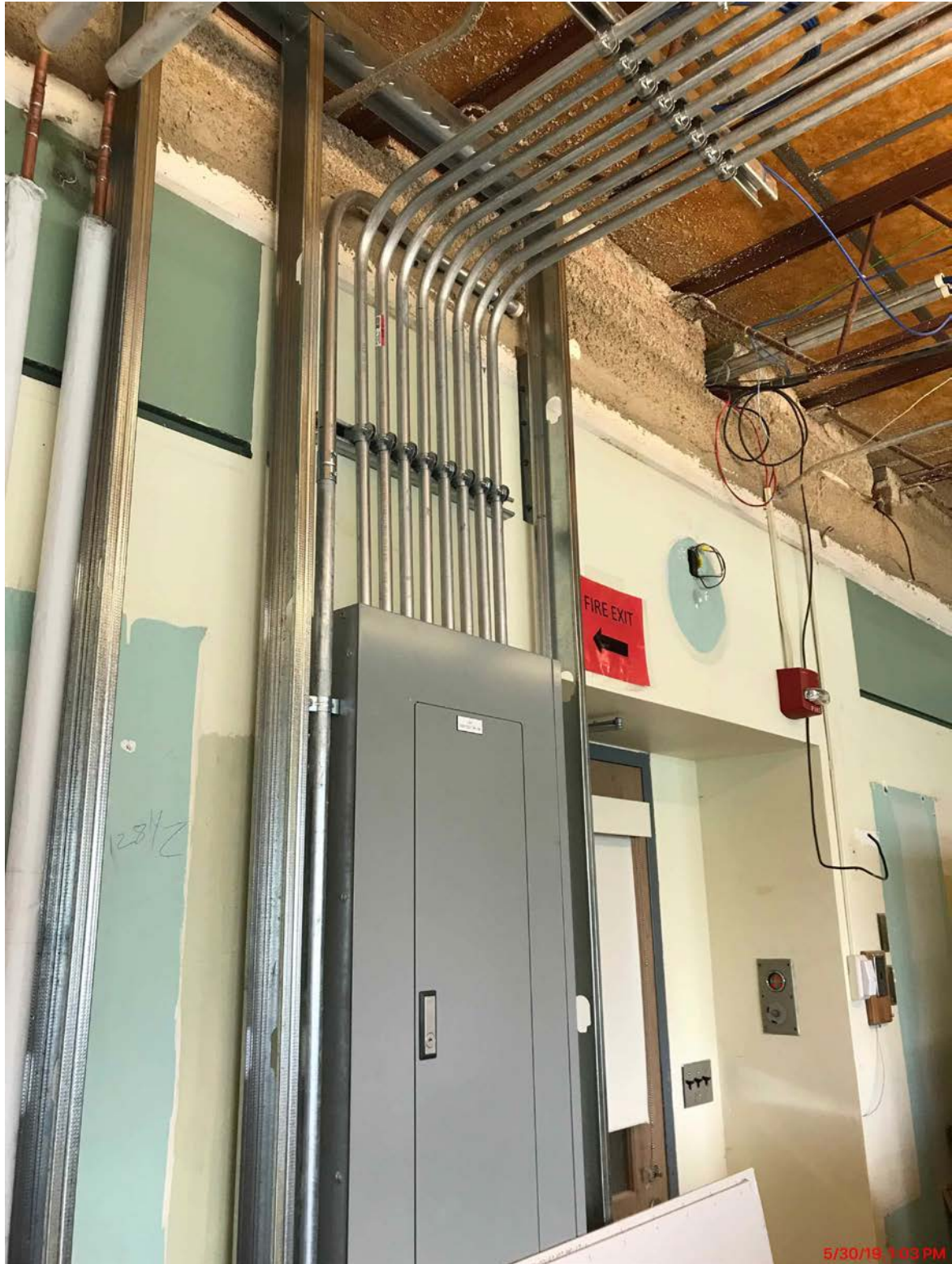
Upgraded Electric Installed in Family Consumer Science Room
