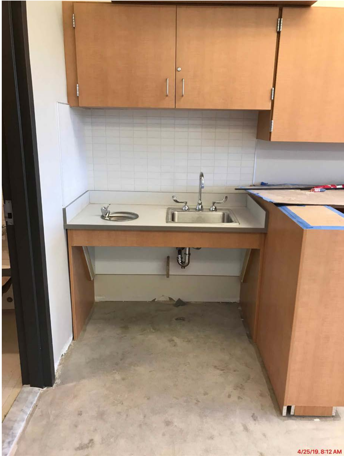
Sinks and Bubblers installed in Eight Elementary Classrooms
