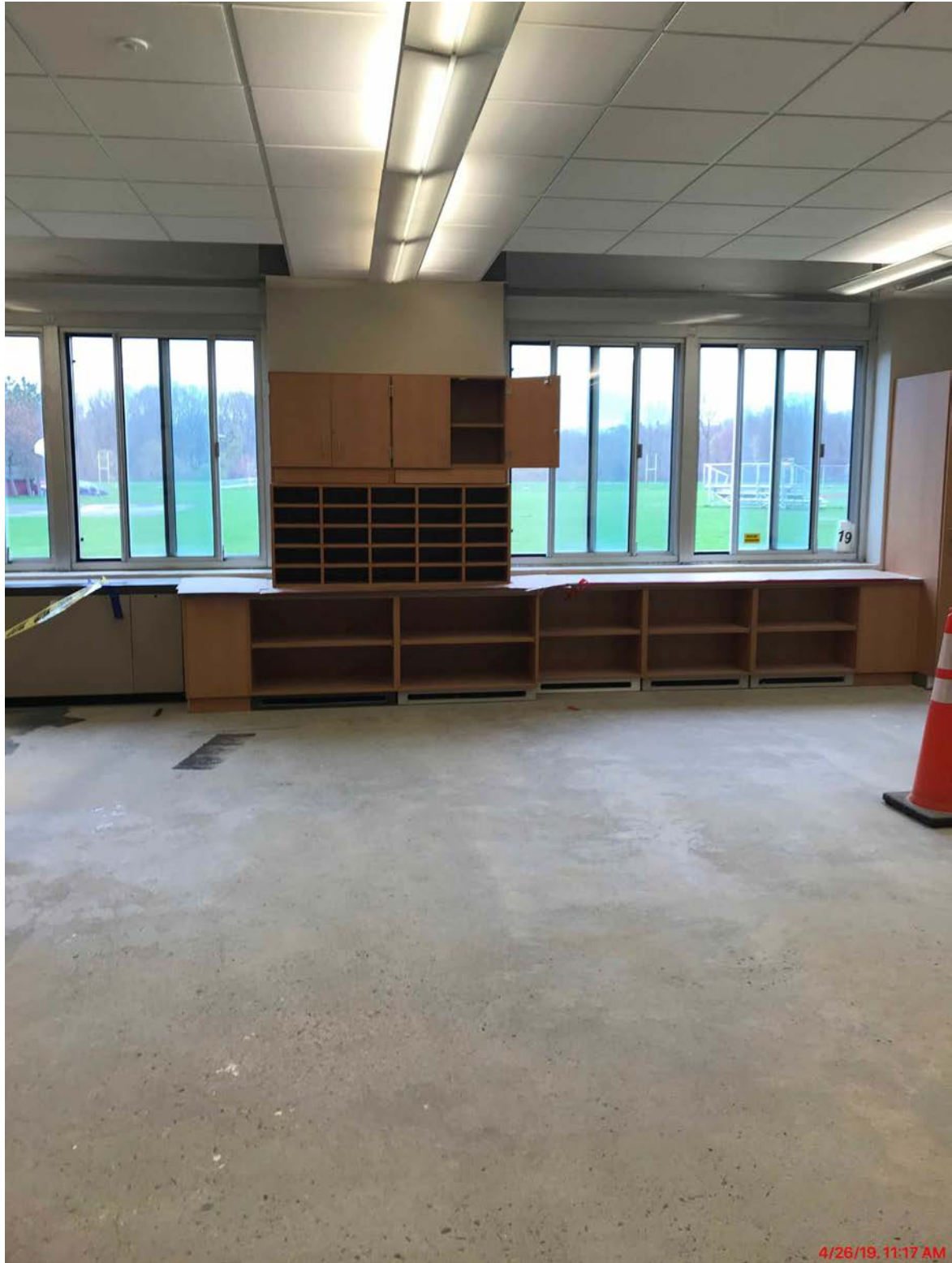
Chrome Book Storage Cabinets Installed in Eight Elementary Classrooms
